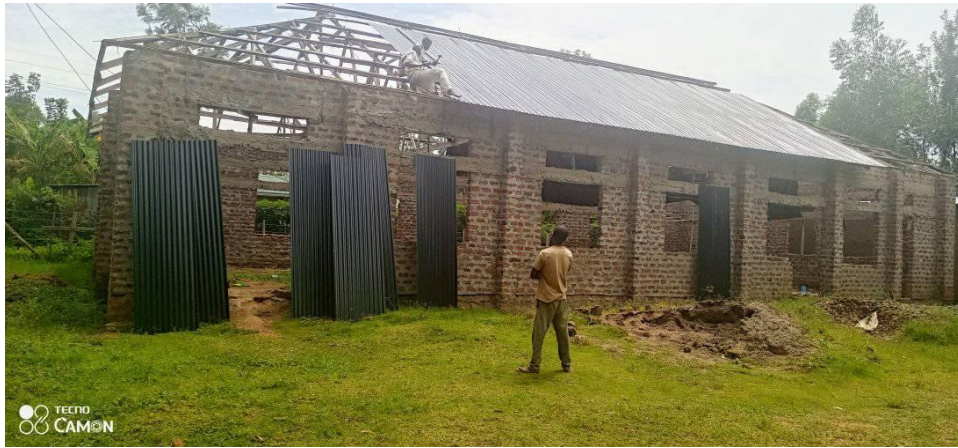
Remember this is the first church where the youths made all those bricks. Now it is getting a nice roof.
